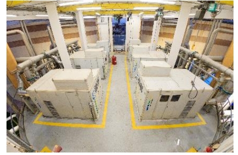
Biogas compressor room (1,361m³/h)
